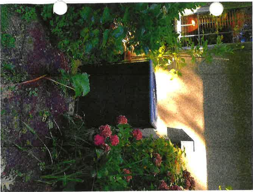
Looking at condenser
