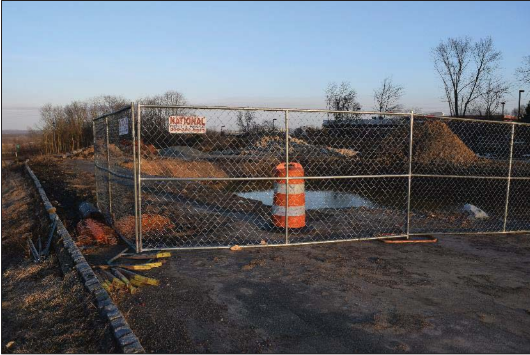
Photograph 5: Existing principal building foundation void.
