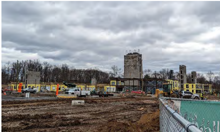
FIGURE 6: CONSTRUCTION OF THE FIRST MULTI-FAMILY, MIXED-USED STRUCTURE DURING THE FIRST PHASE OF DEVELOPMENT (1/26/2023).
